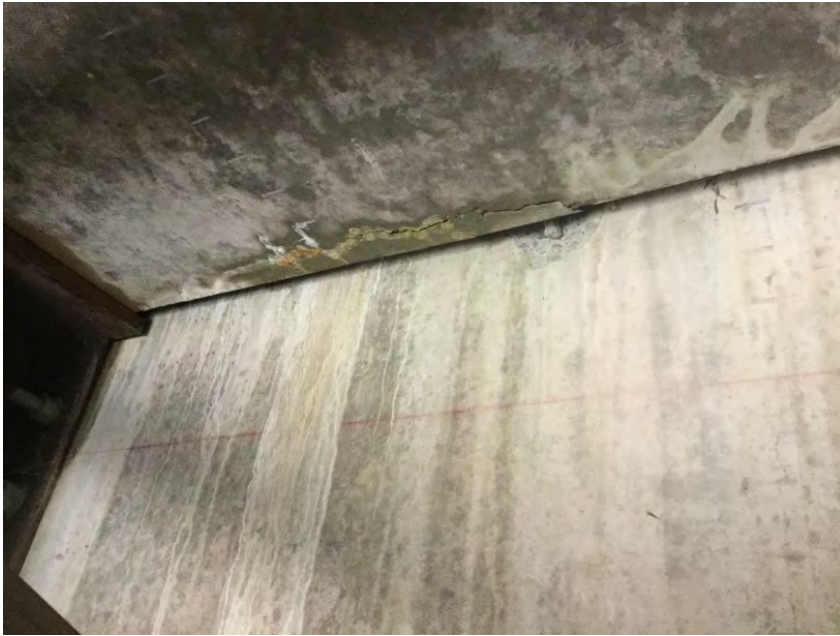
Minor damage noted to underside of panel 1 right bank
