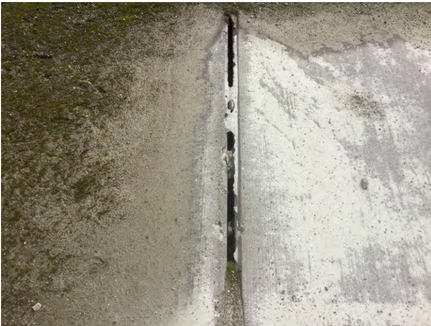
Deck seals all failed
