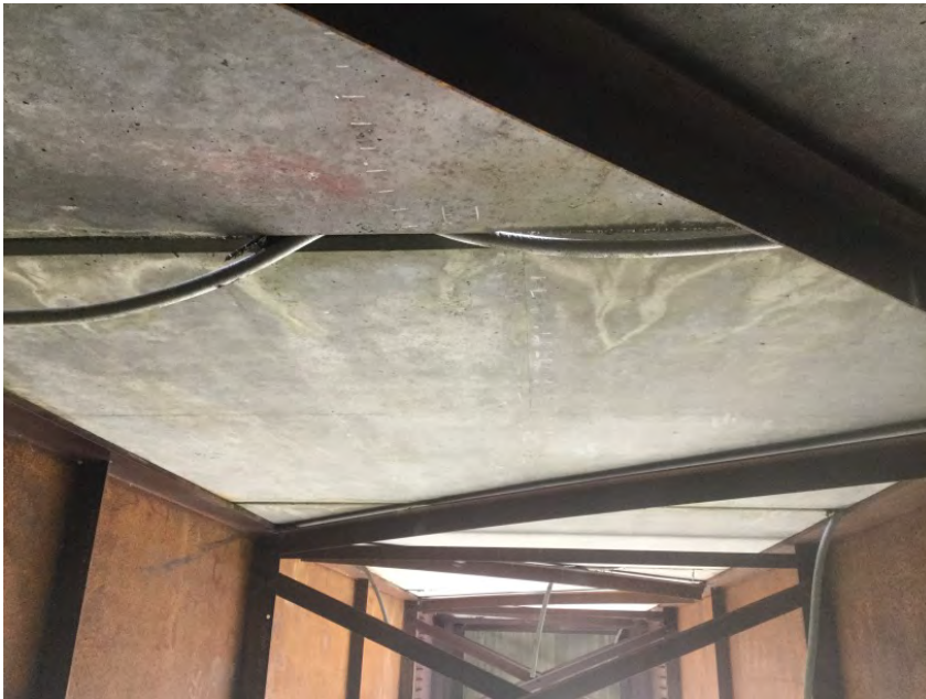
Foam backing coming out of all deck joints
